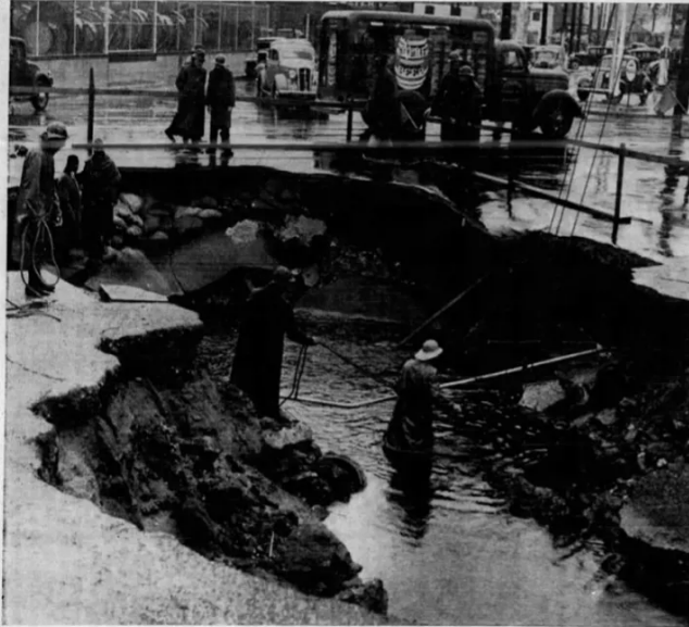
CAVE-IN —Storm-weakened area at intersection of Eighth and Alameda Sts. collapsed at height of gale which deluged Southland with heaviest September rain on record. Times photo
